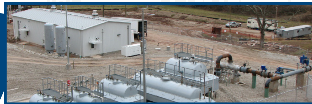
Dominion: Spruce Run Compressor Station
