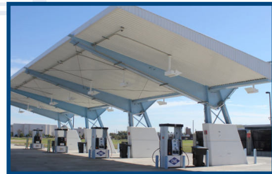
City of Bossier: CNG Fueling Facility.
